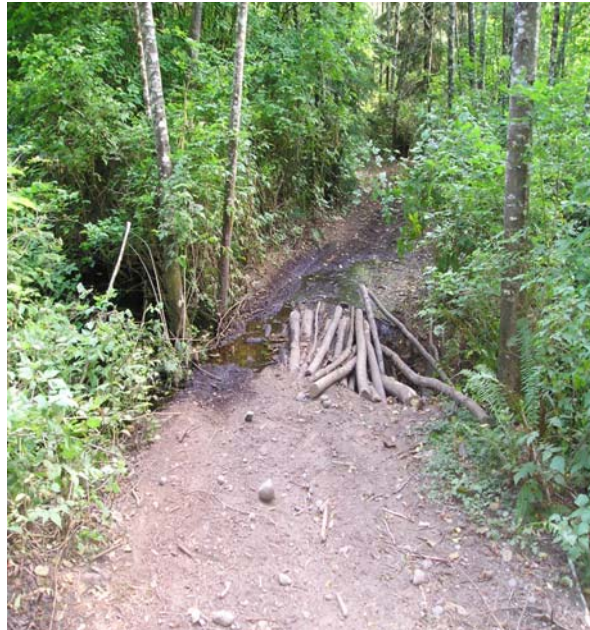
Section IV trail crossing Bear Creek Tributary, June,2003; crushed culvert and logs that were blocking stream flow were removed July, 2003.
